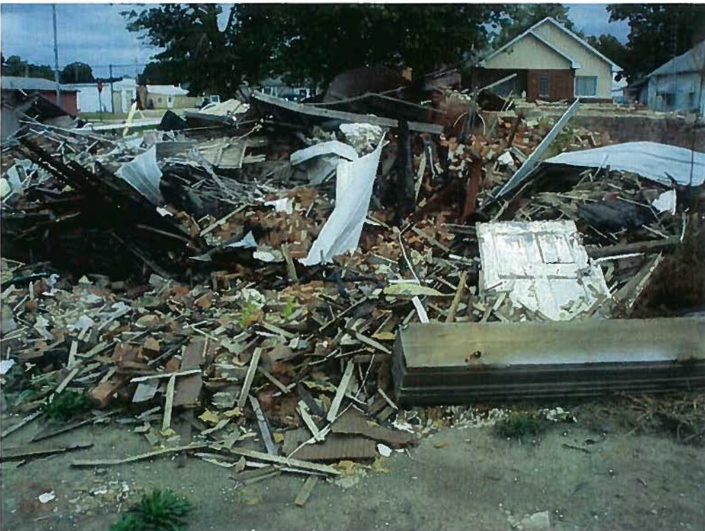
Date: September 16, 2010 Time: 11:35 a.m. Direction: N Photo by: Charlie King Exposure #: 012 Comments: The south side of the demolished buildings.
